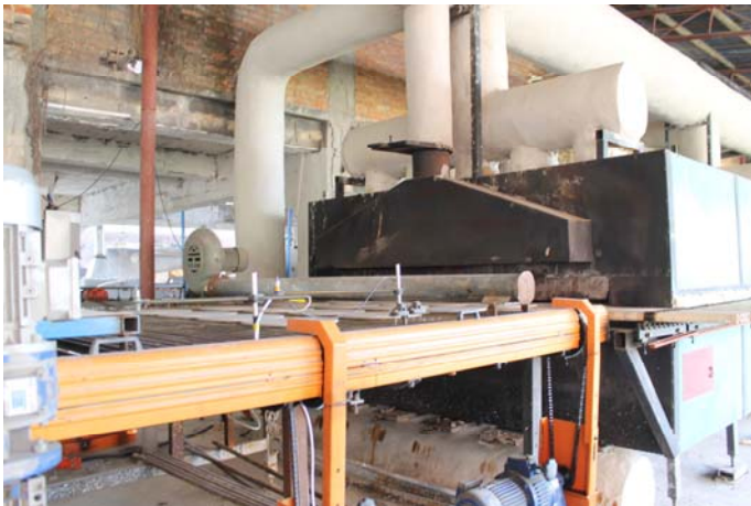
Fire in the roller kiln
